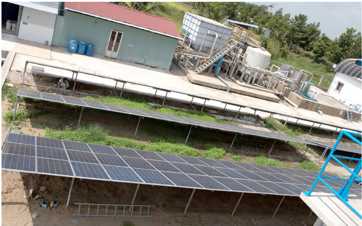
Solar power system installed at the centralized water supply system in Thanh An, Thanh Thang, Thanh Loi commune, Can Tho province
