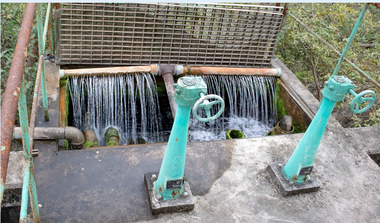
Filtering tank of water plant Hoa Thuong, Thai Nguyen province
