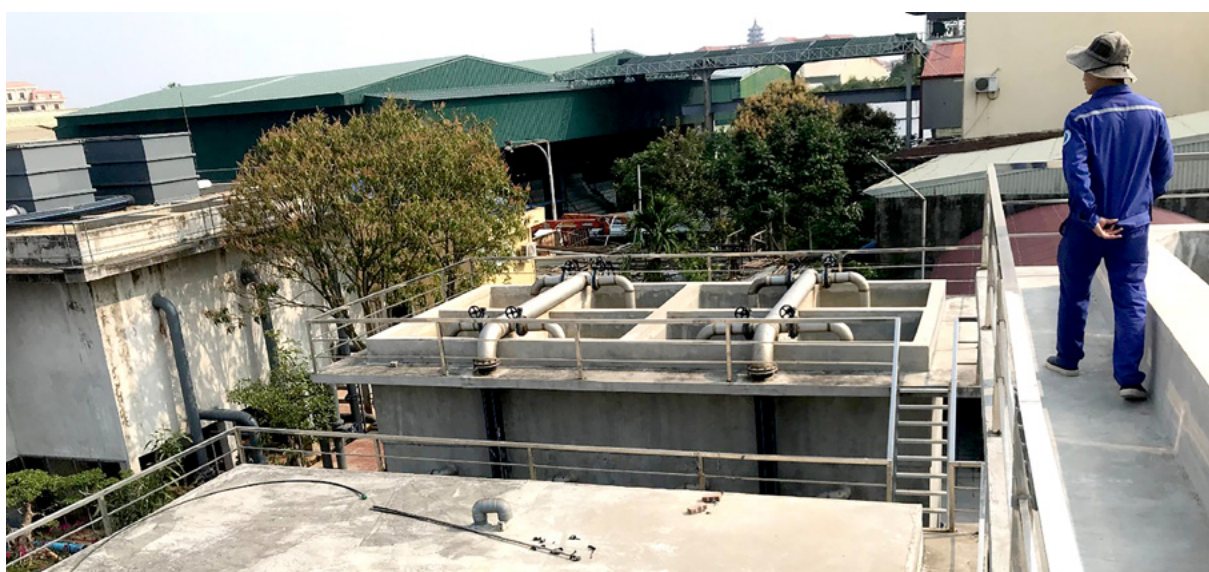
Water treatment area at Xuan Truong Water Plant, Nam Dinh province
